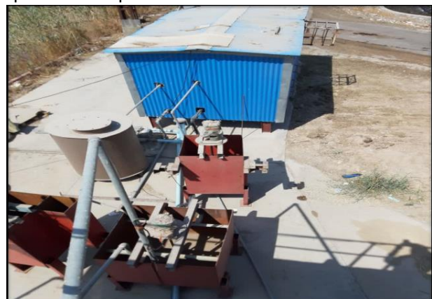
Fig.1. Physical and chemical purification units in pilot
